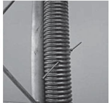
Figure 1-19. While an antenna system could be faulty for any number of reasons, poorly installed connectors, dented/damaged coax cables and defective antennas tend to dominate the failure trends.
