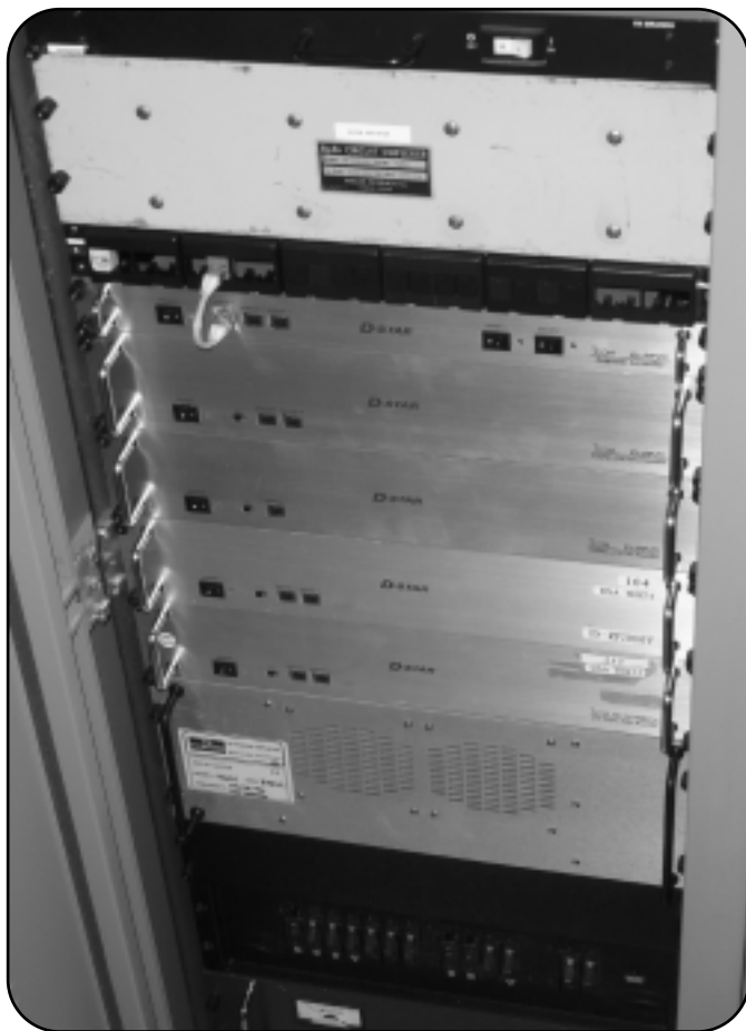
Photo C. The K5TIT rack of D-STAR gear includes (in order, starting near the top of the rack) a D-STAR repeater controller, 1.2-GHz voice repeater, 1.2-GHz data radio, 146-MHz voice repeater, and 446-MHz voice repeater. (Photo courtesy of Jim McClellan, N5MIJ)
